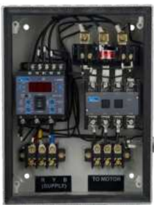
Interior View of MD Starter+ DOL Starter
