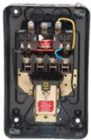
Interior View of MK1 DOL
