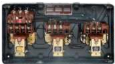
Interior View of MK2 SASD
