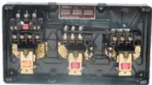
Interior View of MK1 SASD
